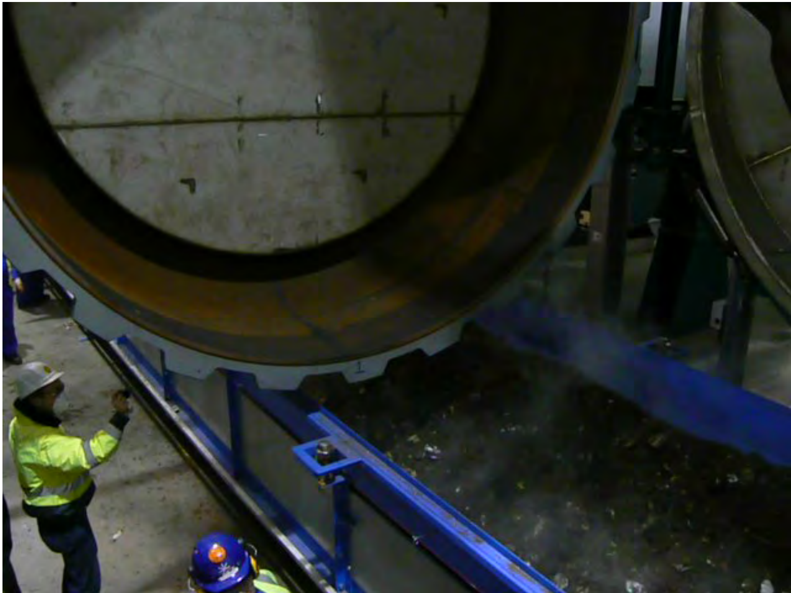
Rotoclave® Vessel Discharge Conveyor moving processed Materials to the Separation Staging Walking Floor
